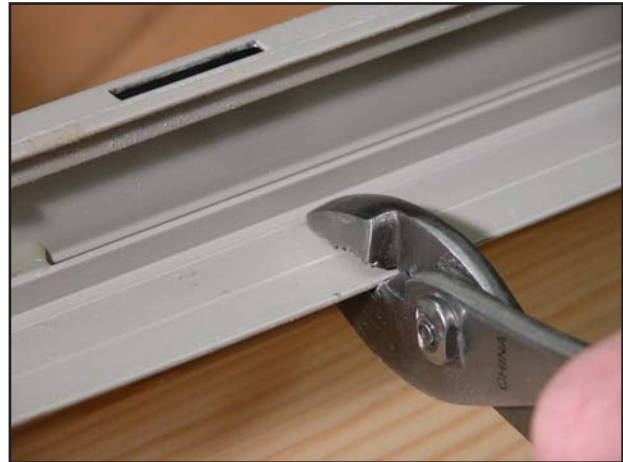
Snap off nail fin from top of door frame and bottom of window.
